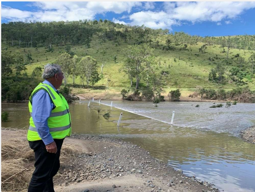
Figure 11. Former Chair of the LDMG (Cr Graeme Lehmann) inspecting damage post the Feb-March 2022 Severe Weather Event (March 2022)
