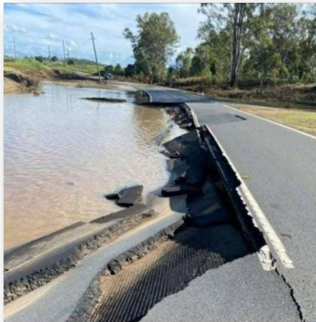
Figure 5: Damage on the Brisbane Valley Highway south of Geoff Fisher Bridge from the Feb-Mar 2022 Severe Weather
